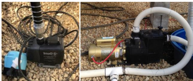
Figure 8. Both submersible pumps and centrifugal pumps can be used to circulate nutrient solution in the plant production pond. (Chris Mullins, Virginia Cooperative Extension)
