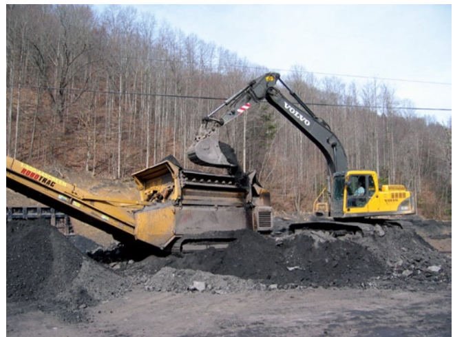
Figure 9. Reprocessing and removing older refuse materials, including pre-SMCRA abandoned mine land piles, is becoming increasingly common in southwestern Virginia, both for the purpose of salvaging marketable coals and for environmental remediation. When the surface materials of these older piles are sufficiently weathered to enable them to support vegetation, separating and retaining these materials for use in reclamation can save money and it can reduce or eliminate the environmental disturbance required to obtain soil cover that otherwise would be needed to restore the area.
