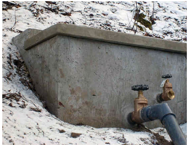
Figure 2. A properly sealed spring box will prevent surface water, insects and small animals from gaining access to the spring. Source: http://aquariuspump.com/springbox.aspx .
