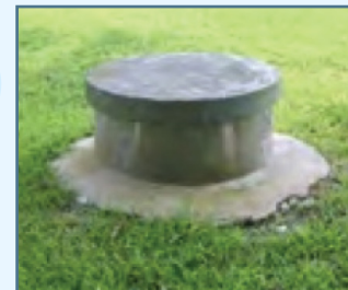
Bored well with sealed concrete cover
