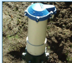
Drilled well with proper casing and secure sanitary well cap
